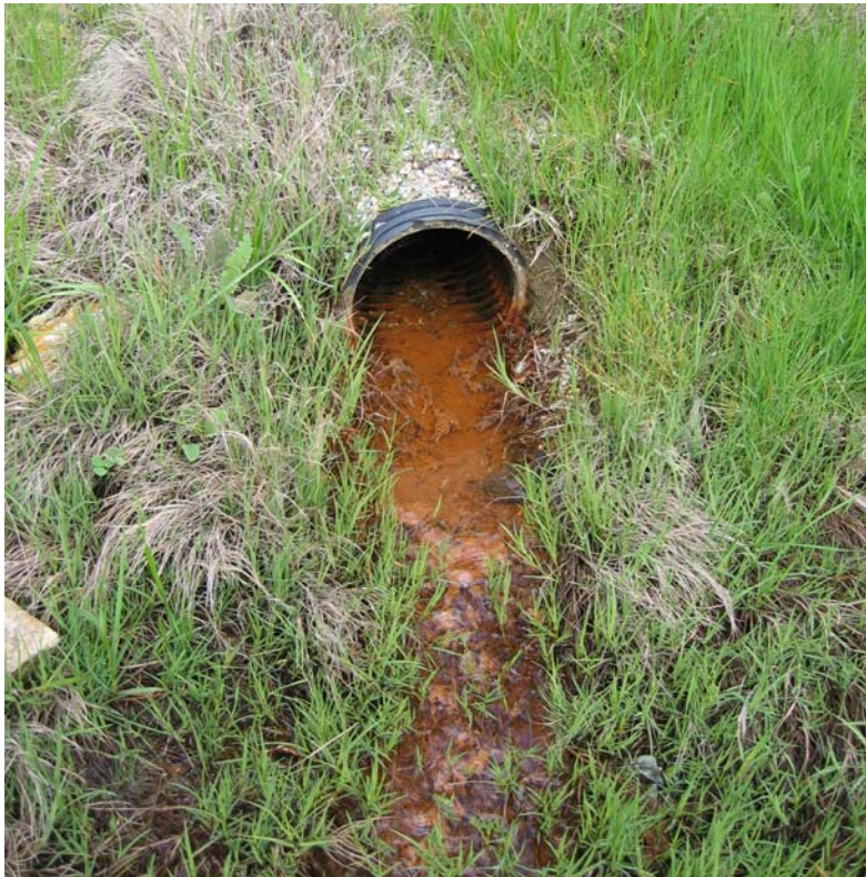
Figure 7. One of two 8-inch plastic culverts that discharge fresh water from the road fill onto Spring 3. The grass in the foreground is Distichlis spicata .
