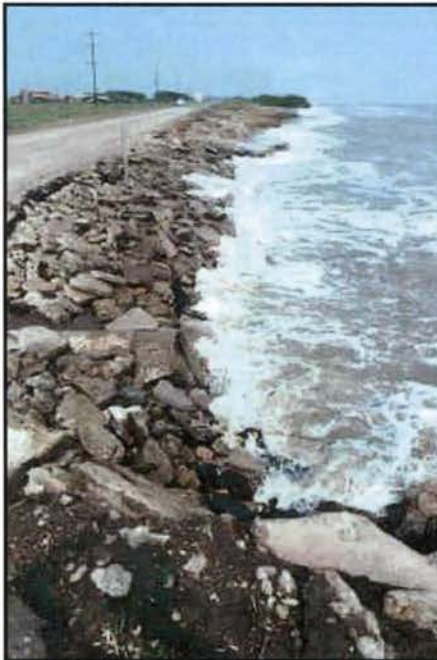
Erosion along LA 82 just west of Holly Beach (May 1991)
