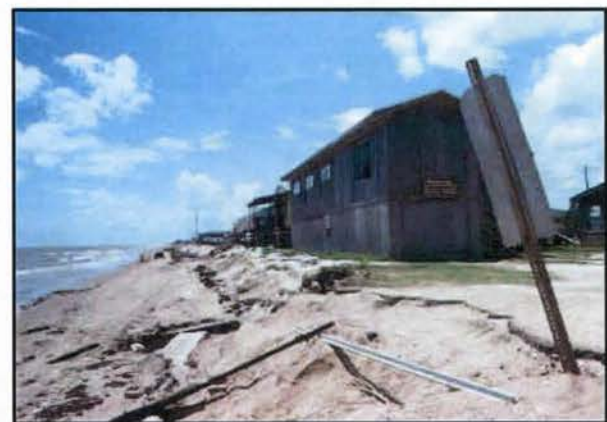
Constance Beach west of Holly Beach. Note erosion before Hurricane Rita (August 1991)
