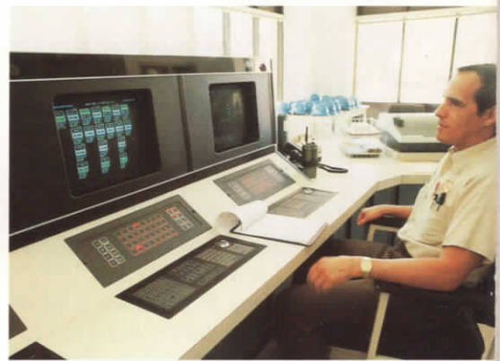
Unit 3's state-of-the-art control room permits continuous monitoring of the facility's operation.
