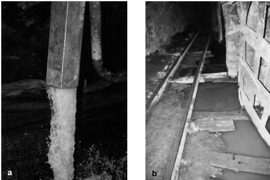
Fig. 4. Acidic mine water management: a – underground water pumped to the main adit, b – water transported by the underground channel
