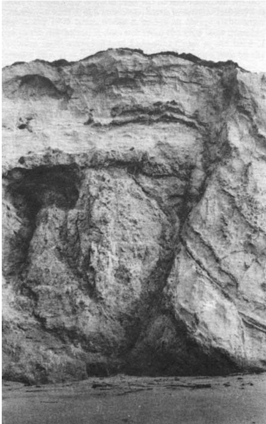
Photo 27. Reverse fault in the sea cliff near Kehoe Ranch. Laird Sandstone has been displaced against granitic basement rock.
