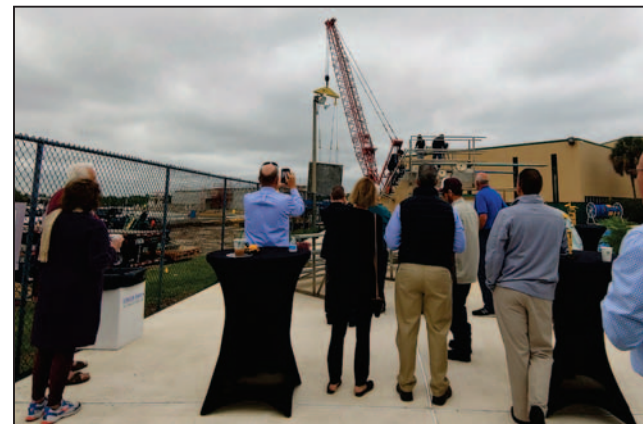
PHOTO BY STEVEN RYZEWSKI Onlookers watch as a prefabricated wall is raised into place during a "Tilt Up Viewing Party" for the Chain of Lakes Field House.
