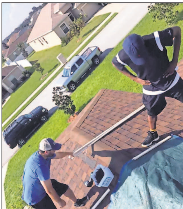
Polk State College Basketball team helped repair and tarp rooftops after Hurricane Irma.
