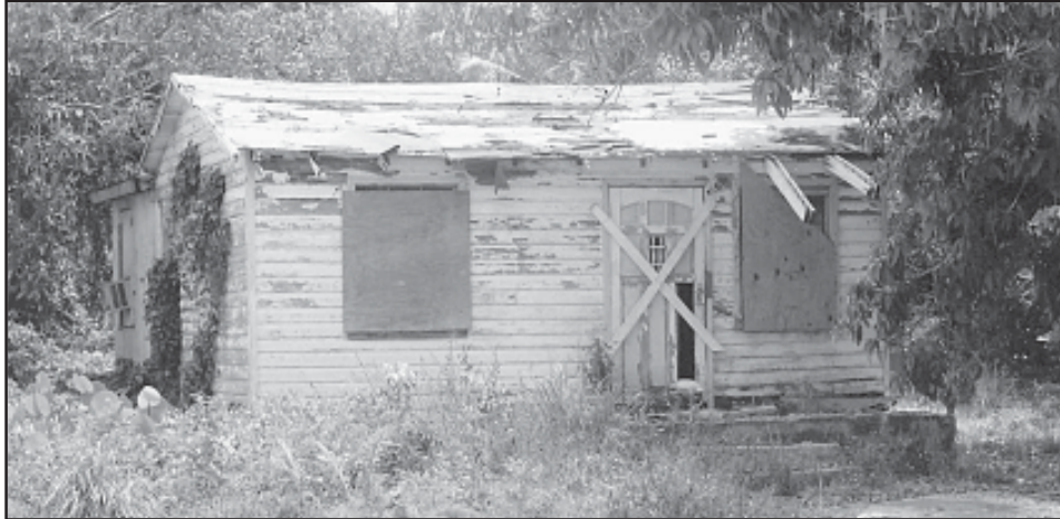
This is one of the dilapidated buildings that mar our town. The Ministry of Works will be tearing them down. They have already notified owners preparatory to cleaning away the eyesores.
