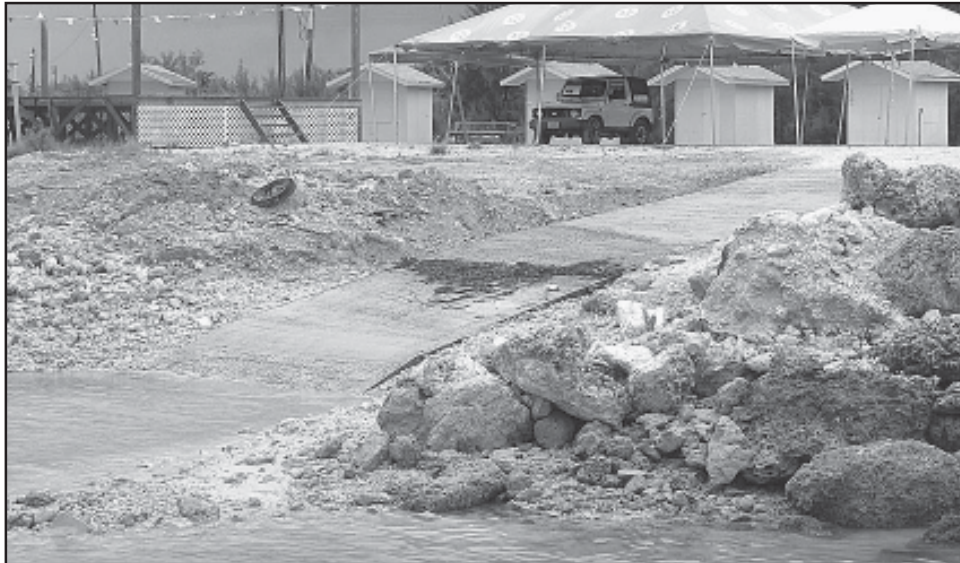
The Marsh Harbour Town Committee was allocated $25,000 for small capital projects this past winter. Two projects that they undertook was to build the wood extension on the dock and to build a boat launching ramp at Goombay Park. The only other ramps in Marsh Harbour are both private. The one most used is at Iron Point west of Snappas and vehicles launching or hauling boats there cause traffic problems. Another improvement to Goombay Park is a wooden walkway joining the stalls which also provides seating for those attending events at this location.
