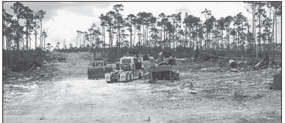
Preparation of Phase II of Central Pines Estates is underway. Roads are under construction and the area will soon be ready for utilities to be put in. Phase I is completely sold out and those reselling their lots in that area are selling for several times the original cost of the lots.
