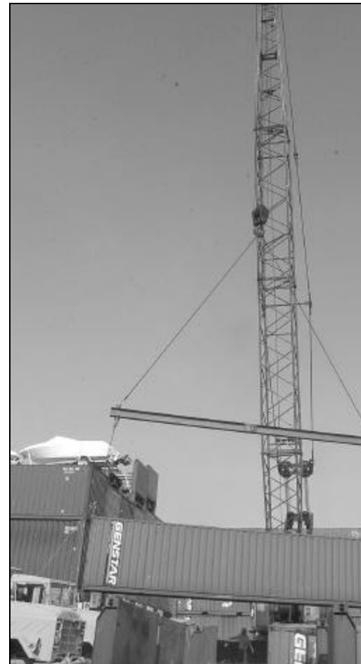
A heavy-duty crane is used to hoist all secured cargo from the barge.
