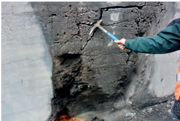
Figure 1. Ghost rock in the Gauthier-Wincqz Quarry in Soignies, Belgium. The limestone, a massive Tournaisian (Mississippian) 'encrinite' was partially dissolved, especially its micritic part. The larger remains of the crinoid fossils give a granular aspect to the 'ghost'. Inside the ghost-rock, remains of unaltered or less altered limestone are observed, e.g., behind the hammer.
