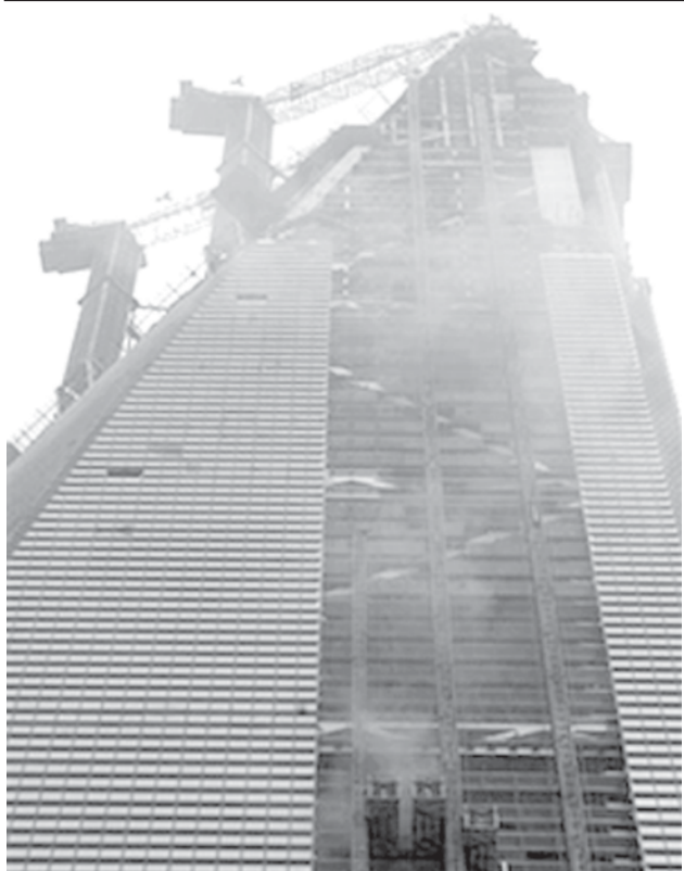
Smoke billows from the World Financial Centre in Shanghai, China, on 14 Aug, 2007. Fire broke out Tuesday at the site of China’s future tallest building, although there were no immediate reports of injuries or deaths. —INTERNET
