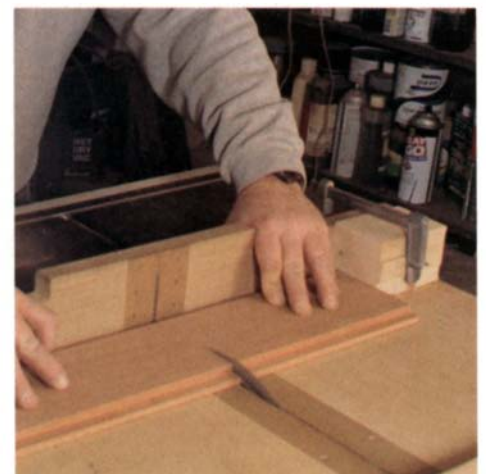
Cut the rabbeted sides apart and to length on the table saw. Use a stop block to ensure consistent lengths.
