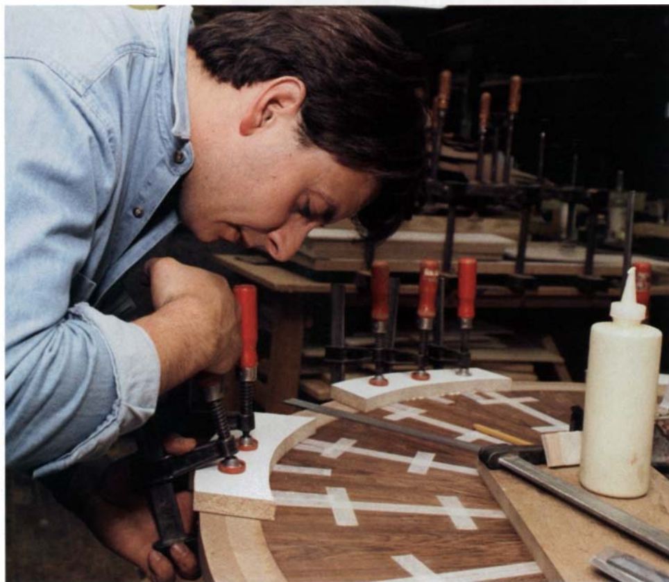
Angle the clamp out, so it forces the crossbanding inward when you apply pressure.
