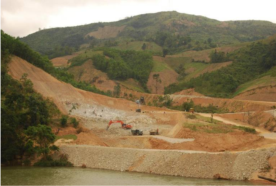
The construction of Dakrong 2 hydropower station in Dakrong Commune ©Nguyen Thi Hanh Tien
