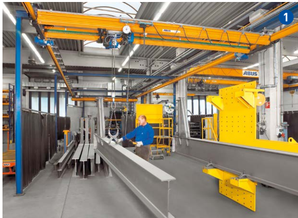
1: ABUS ZHB-X raised up double-girder crane
