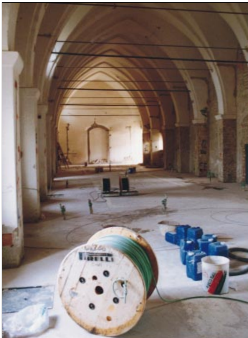
The installation of Pirelli's Afumex power cables in the church of S. Francesco in Assisi.
