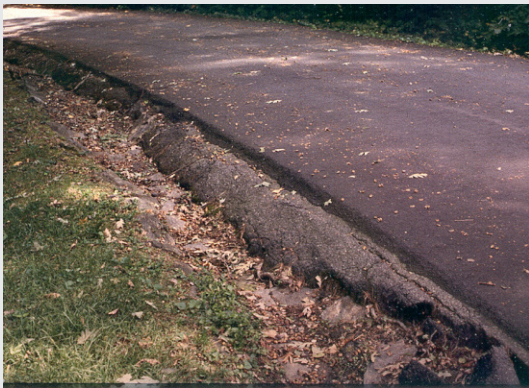
(Above) Asphalt was layered on The Circle, so much that it covered much of the original stone swale.
