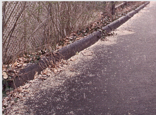
(Above) Rolled asphalt curbing was installed on the upper parts of Cherokee and Canterbury Roads.
