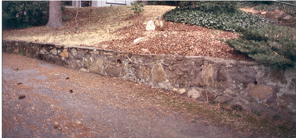
The primary form of wall used in Albemarle Park is the low stone retaining wall, rarely exceeding 3' in height. It is used to effect a change in grade where an unsupported
