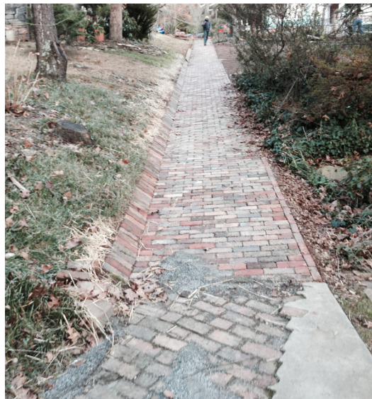
Asphalt covering existing brick was removed and original brick was reinstalled on Hillside Walk in 2013.
