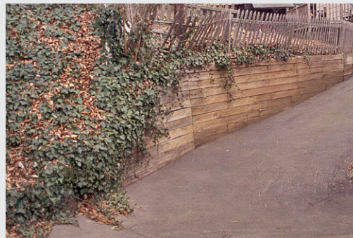
A relatively recent retaining wall constructed with wood beams. (The visual appearance of this wall could be improved by planting and allowing vines to grow up and cover it.)
