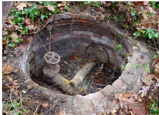
(Above) Steam valve in a brick-lined pit behind Manzanita Cottage. This controlled the steam heat coming from the Manor Inn's boiler to several of the cottages up the hill.
