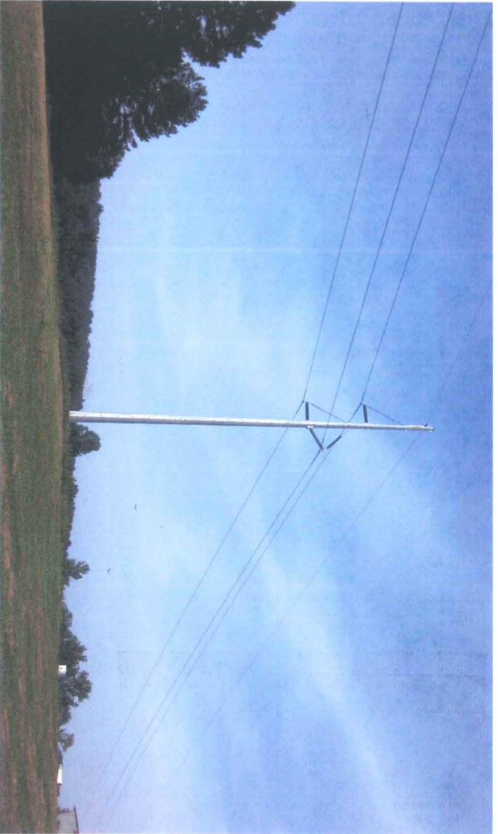
Figure 2. Typical T-Line Pole Configuration.
