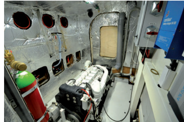
The engine room is equipped with cameras, to keep an eye on the engines from the steering position...
