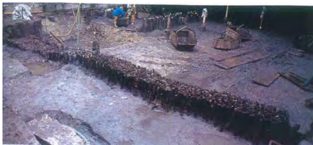
Figure 53a: The oldest foundation piles found recently within the basement of the building of the ex-cinema San Marco .
