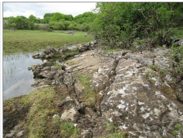
NTSV14_Photo_018_2_FON_01a.jpg 2 Flooded pavement
