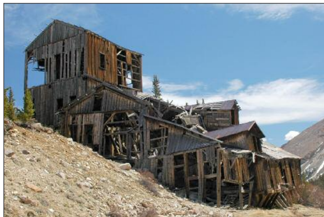
Fig.1 The ruins of an old mine high in the mountains of Colorado.
