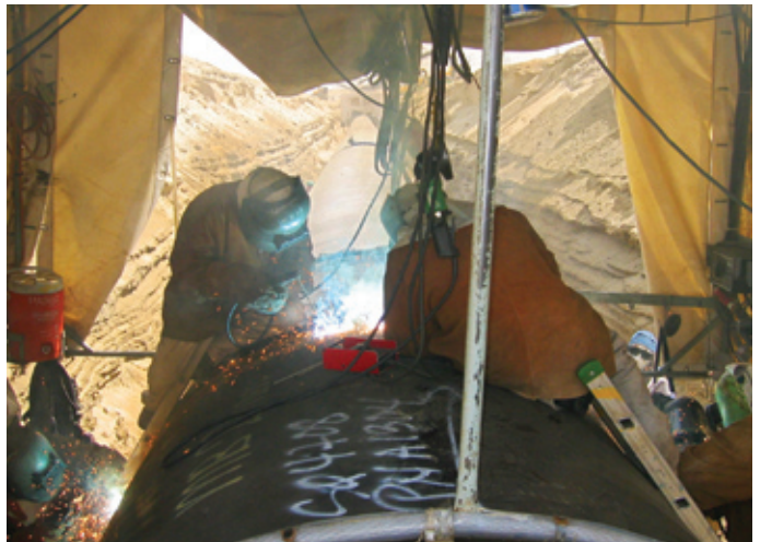
Welders work on a water pipeline in Saudi Arabia using the new electrodes. Photo © BÖHLER WELDING
