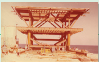
1978 - Egypt - Ras Gharib Shallow water platforms
