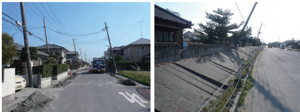
Fig. 6. Liquefaction-damaged district, Hinode, Itako City, including lateral spreading damage of a road (right).
