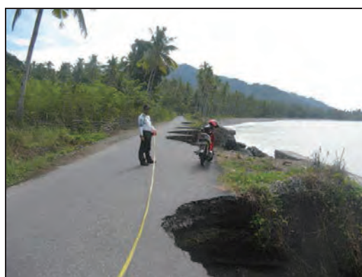
Fig. 27. Indication of creep along the road near to the shoreline
