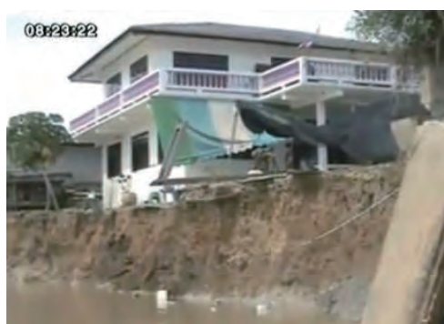
Fig. 14. Bank erosion by overloaded construction.
