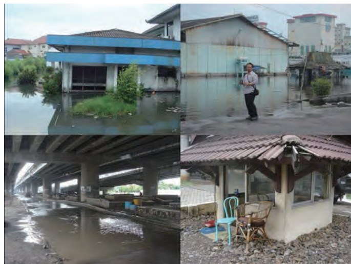
Fig. 22. The land subsidence in Semarang has caused damage to buildings, roads, railways tracks and other items of urban infrastructure.
