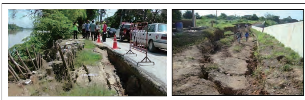
Fig. 13. Bank erosion by running vehicles.
