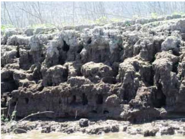
Figure 5.9. Nesting Holes Excavated in the Dam by Loricariids
