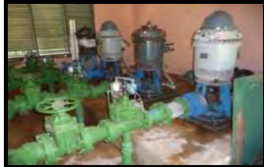
Photo 3.14-4. Maui Well #2 Pump Equipment
