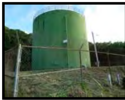
Photo 3.14-6. Carolinas Water Storage Tank (500,000 Gallon Tank)
