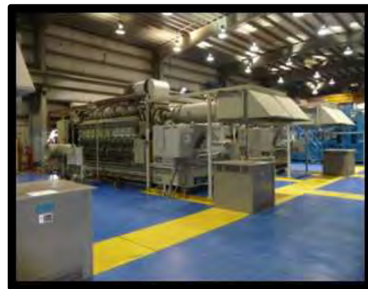
Photo 3.14-1. Power Generation Facility
