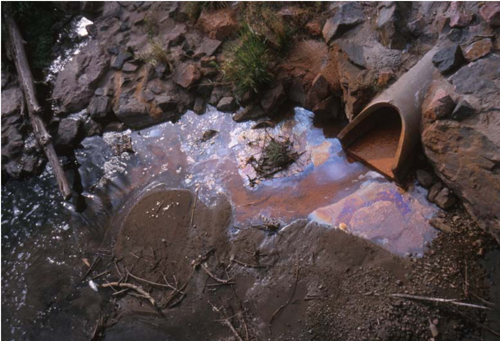
Polluted storm water discharge from a culvert at the pedestrian underpass at Johnson Park. Note dead fish in the lower left of photo.
