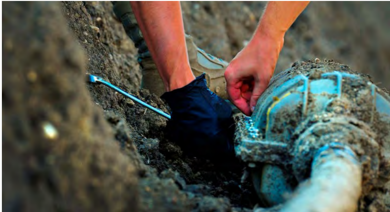
Military personnel splice a cable in the hardened intersite cable system. (Photo credit: Minot Air Force Base)
