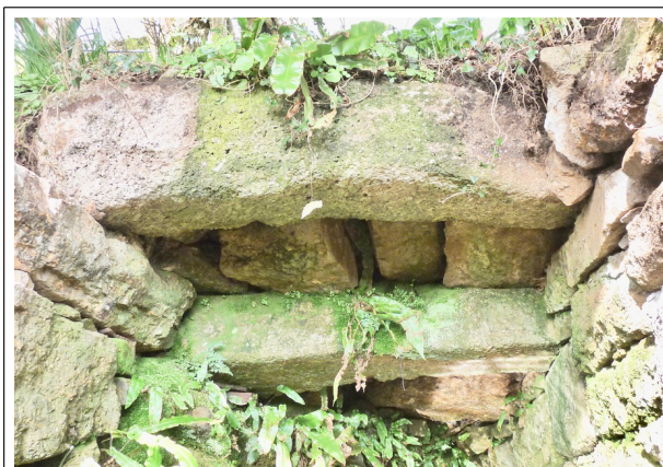
How the roof of the same well was built into the hedge.
