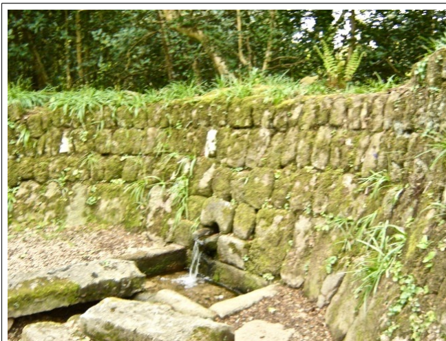
A handsome Cornish hedge around a spout. Unfortunately the original granite slabs are here seen in process of being taken out and an ugly modern grating installed for no apparent reason.
