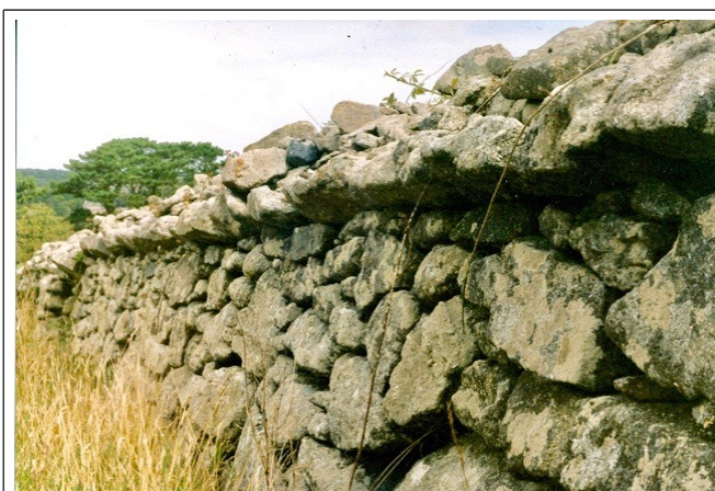
Surviving stone hedge at Godolphin built with a coping on the park side to deter deer from jumping out.
