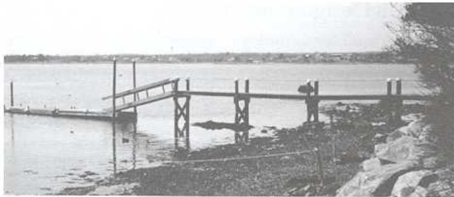
All residential docks in coastal waters have to now be registered with the CRMC.
