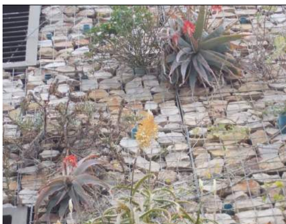
Figure 7: Dry wall of Plant Science Building. Photo: J. Sampson.
