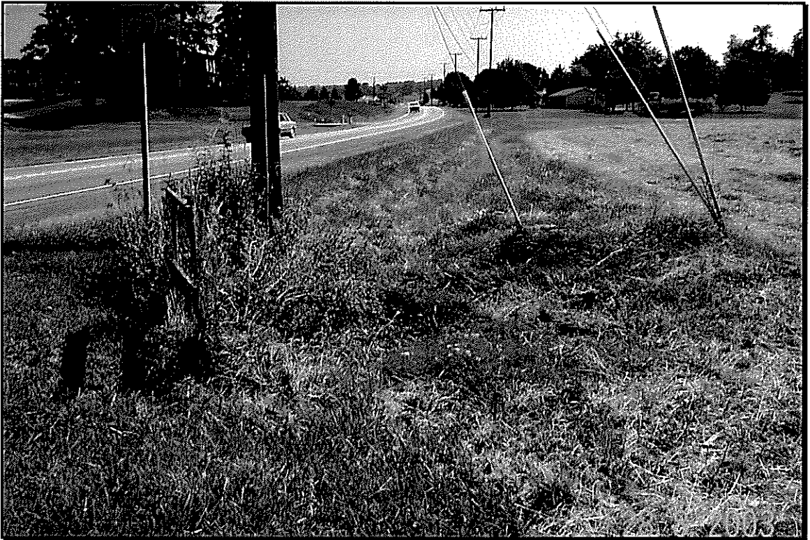
Photo 6. Roadside drainage. This ditch originates near Area 2 in the background. The ditch enters a cross pipe near the utility pole in the foreground.
