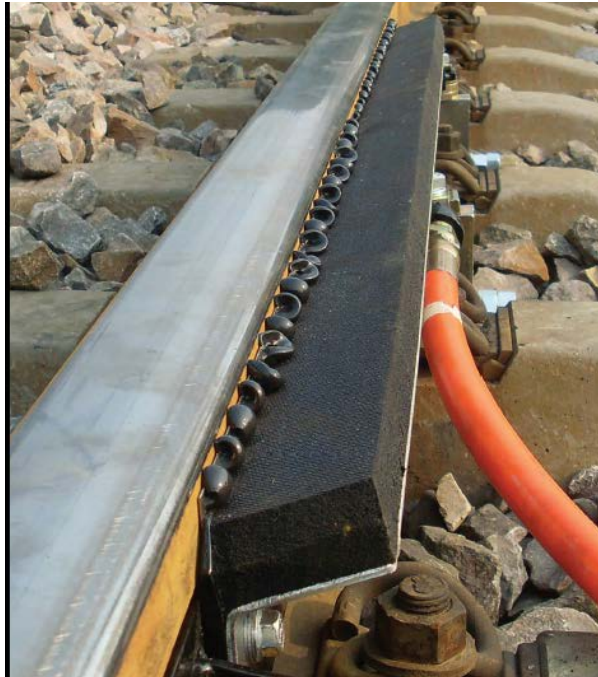
Automatic Wayside Running-Corner Lubrication, LB Foster
