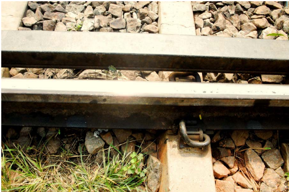
Curve Check-Rail with wide Flange-Way Clearance on a Curve of the SLR Main-Line without any Function
