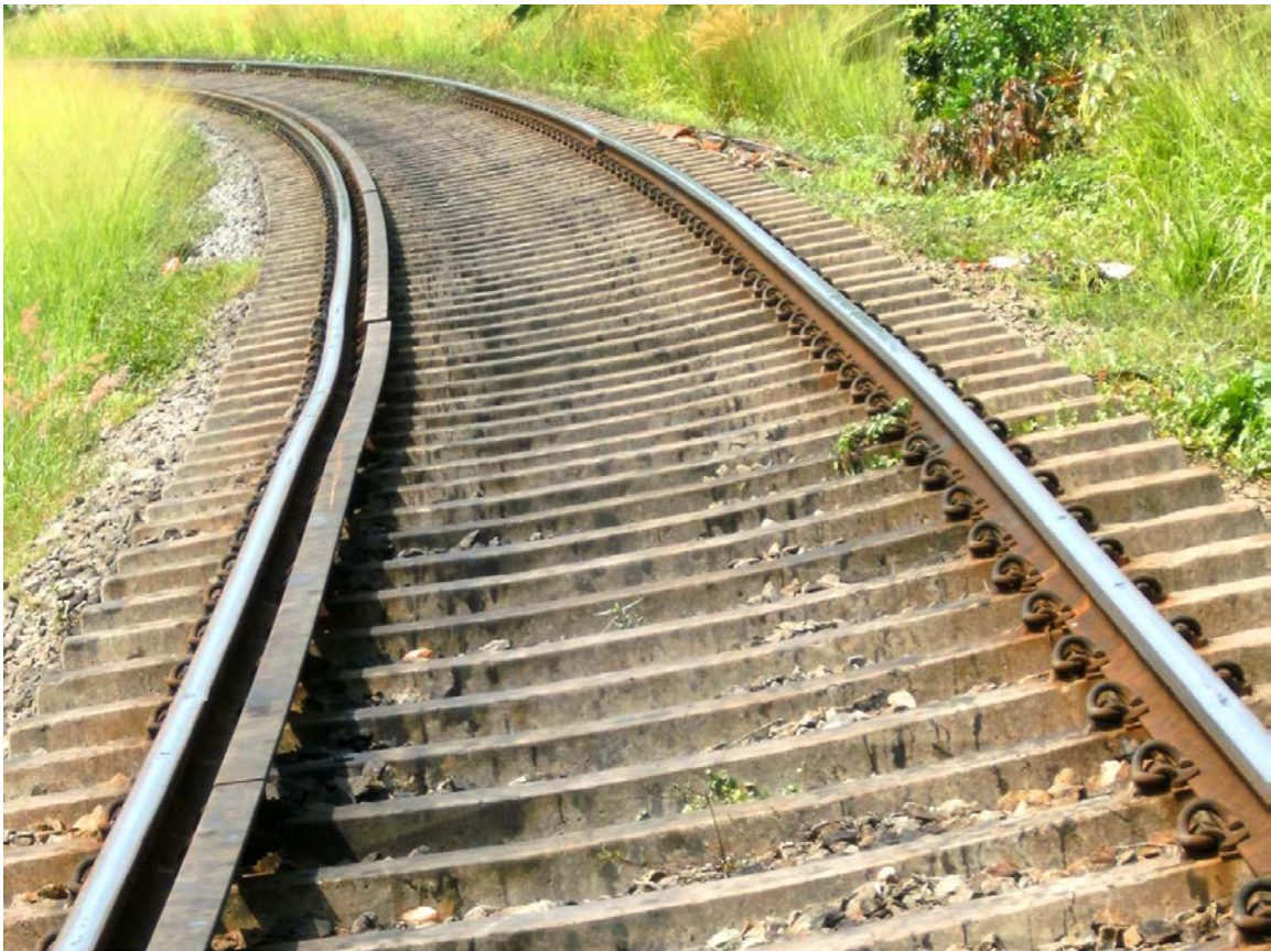
Curve Check-Rail on a Curve of the SLR Short Welded Rail (SWR) Main-Line Track; without any Function
