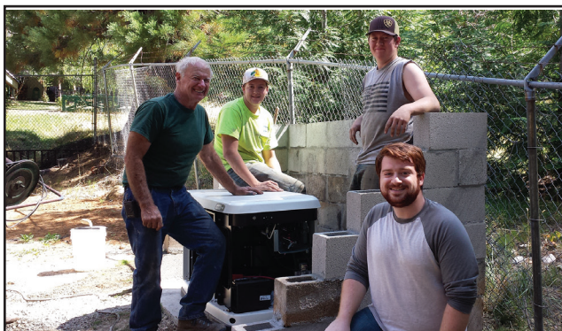
Crew installing backup generator from L to R: Charlie Bridges (Facility and Distribution Mgr), Construction Crew Nick and Ben Thompson and Plant Operator Alec Vrooman
