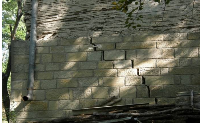
Fig. 2. Foundation Crack (Construction Located on the Surface Associated to the Mine)
