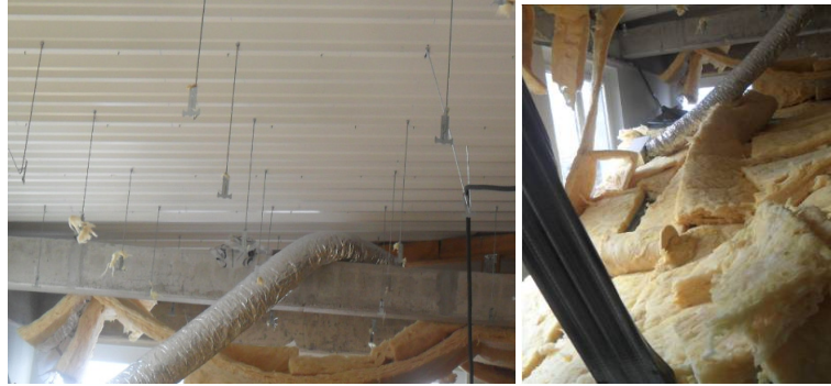
Fig. 1 Infield observed conditions and damages
