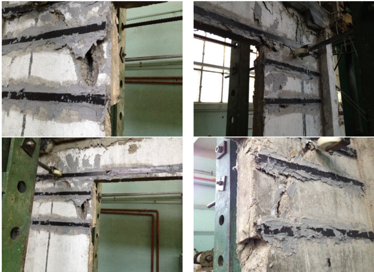
Fig. 6 Failure details of the specimen
