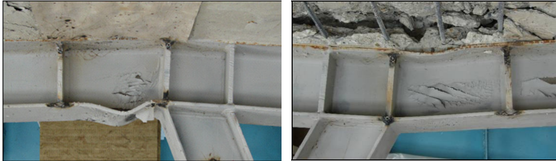
Fig. 7 Dissipative behaviour of the beam without connectors on dissipative zones – left and right side of the link
