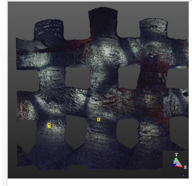
Fig. 6 Highlighting of the ceiling detaching in the rooms 22 to 24, G and H alignments
