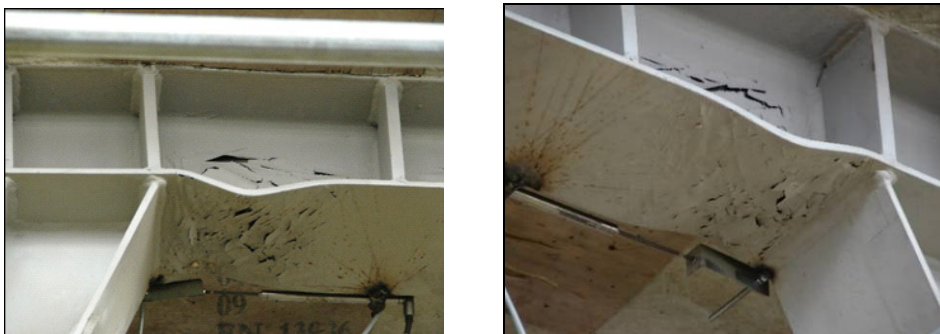
Fig. 9 Dissipative behaviour of the beam without connectors on dissipative zones – left and right side of the link
