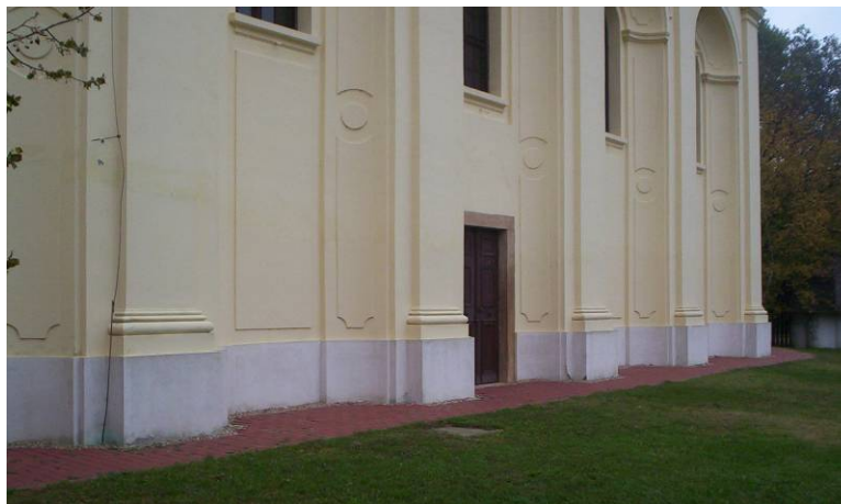
Fig. 2 High level of damp on the outside of the church
