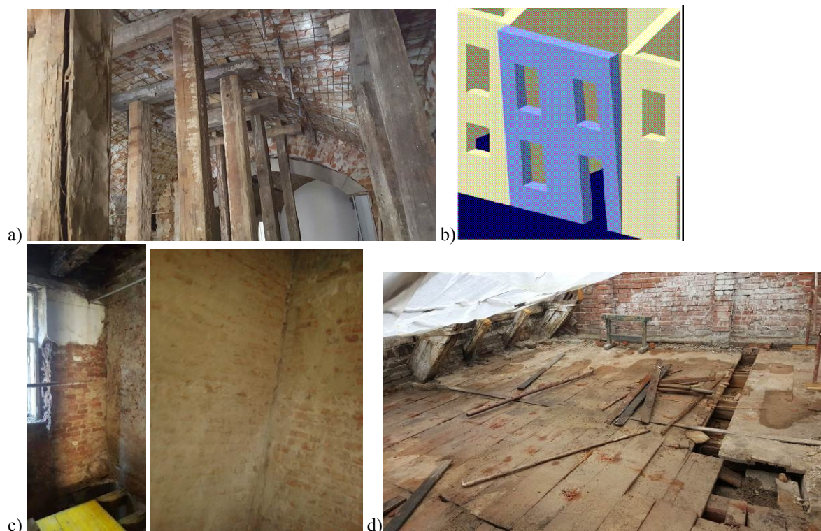
Fig. 4 a) Vault settlement with damages for Sf. Gheorghe building; b) the out-of-plane failure mechanism; c) transversal walls that are not connected to the façade walls; d) ties on the roof structure
