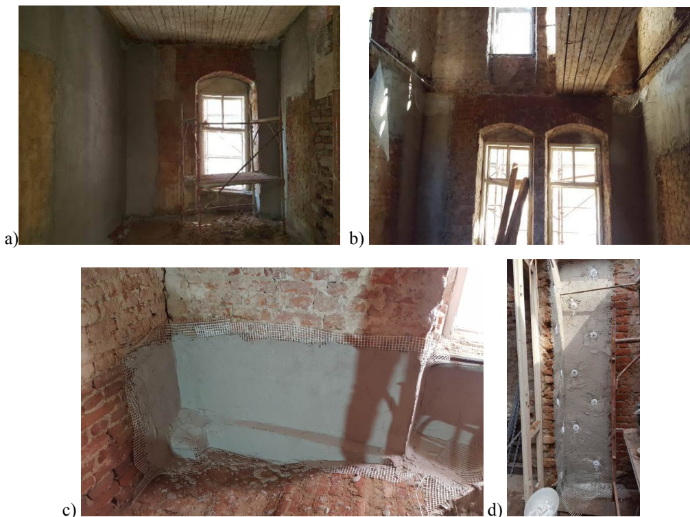
Fig.6 a), b), c), d) The way of putting the reinforcement grids for connecting the façade walls with the interior transversal walls
