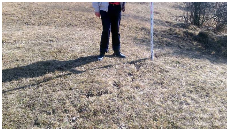
Fig. 8 Cracks on the ground in the planned pipeline area, due to stretching deformation
