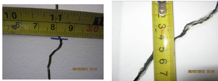
Fig. 2 Measuring transverse cracks in the structure of the old buildings
