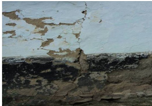
Fig. 3. Crack in the main façade
