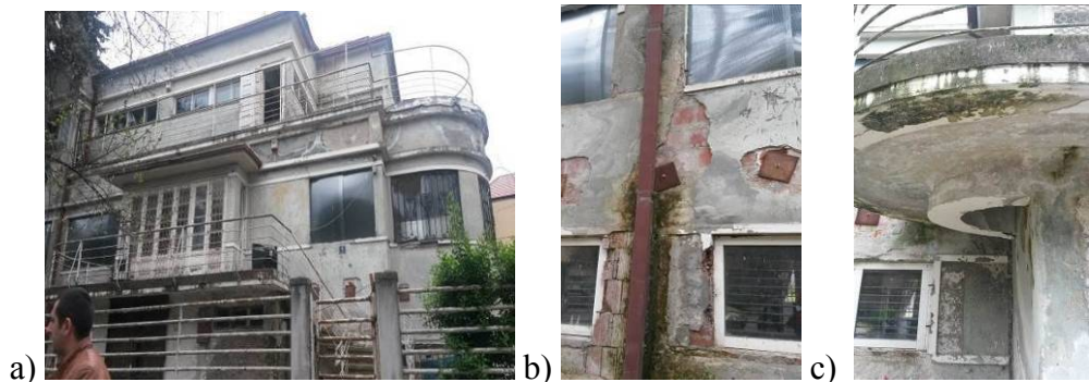
Fig. 1 Degradation of the building facades
