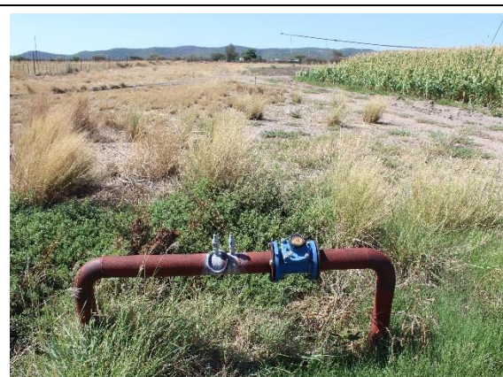
Photo 4-12 Flow meter at boreholes
