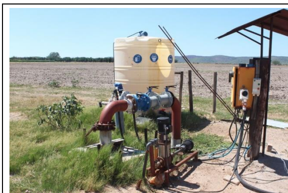
Photo 4-9 Borehole with installed pump and fertiliser reservoir mixing unit
