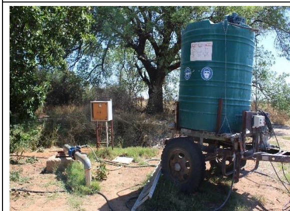
Photo 4-21 Mobile mixing tank
