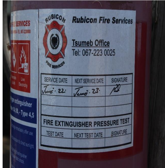
Photo 4-18 Services dates on fire extinguisher
