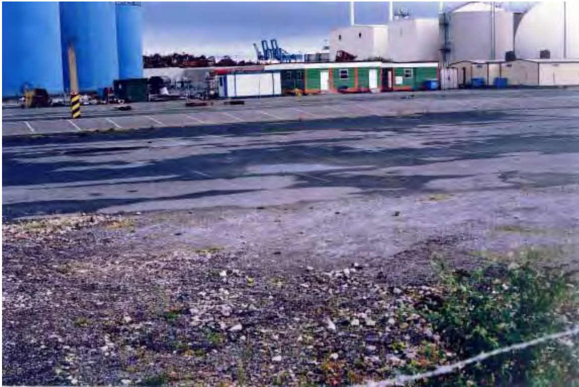
Plate 1. The southern part of the site is a former car-park. Some cracks are appearing in the tarmac surface which provide a niche for plants. View is looking northwards.
