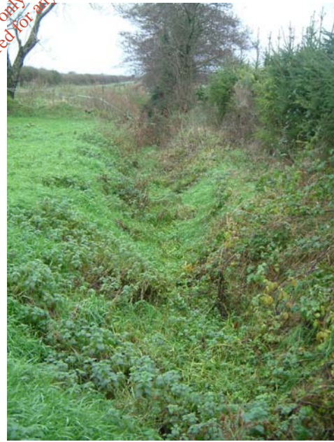
Photo 2.4 Land Drain to Cashen River
