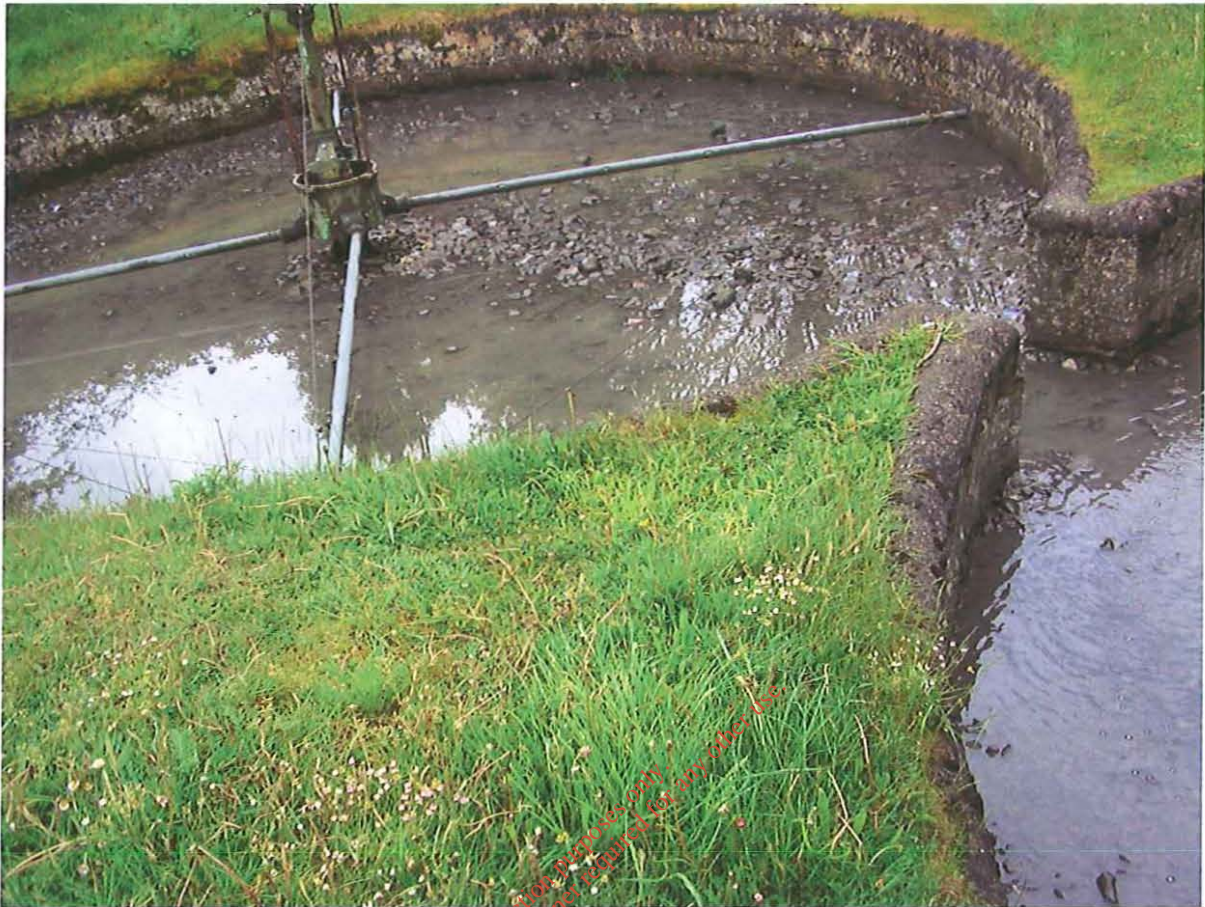
Photograph 2.2 Ponding on the Existing Biological Filters
