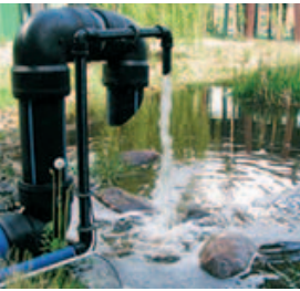
Transfer of rainwater from the cisterns
