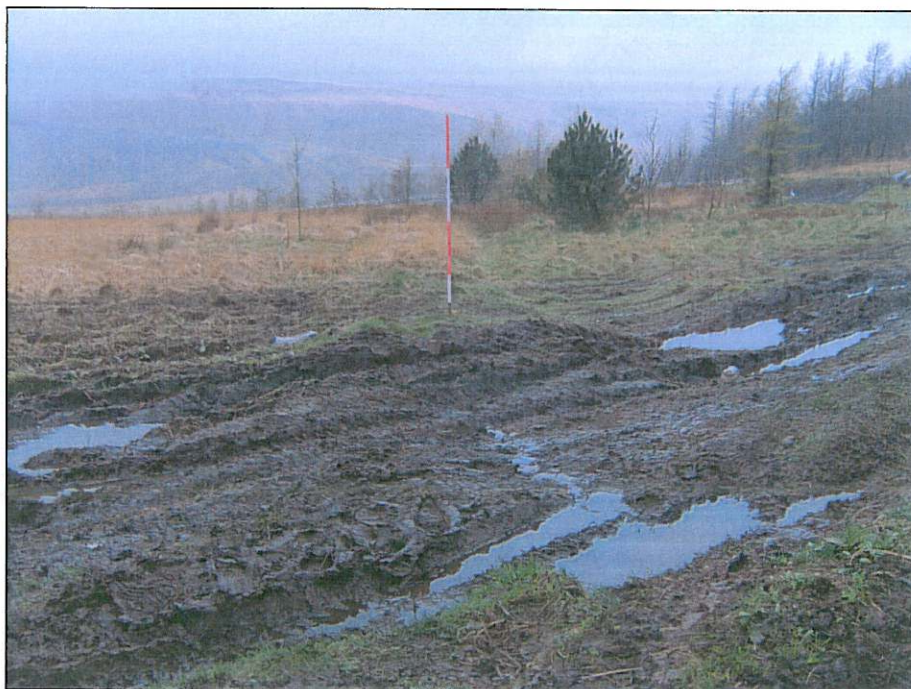
Plate 11: View to west of Bedd Eiddil Dyke (02266.0m) showing damaged area. 2m scale in shot
