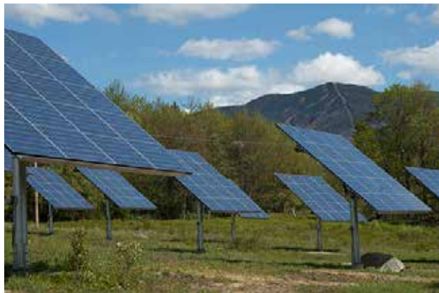
A section of the 35-tracker solar farm at Smugglers' Notch Resort, with the ski trails on Madonna Mtn. in the background. Image: Smugglers' Notch.
