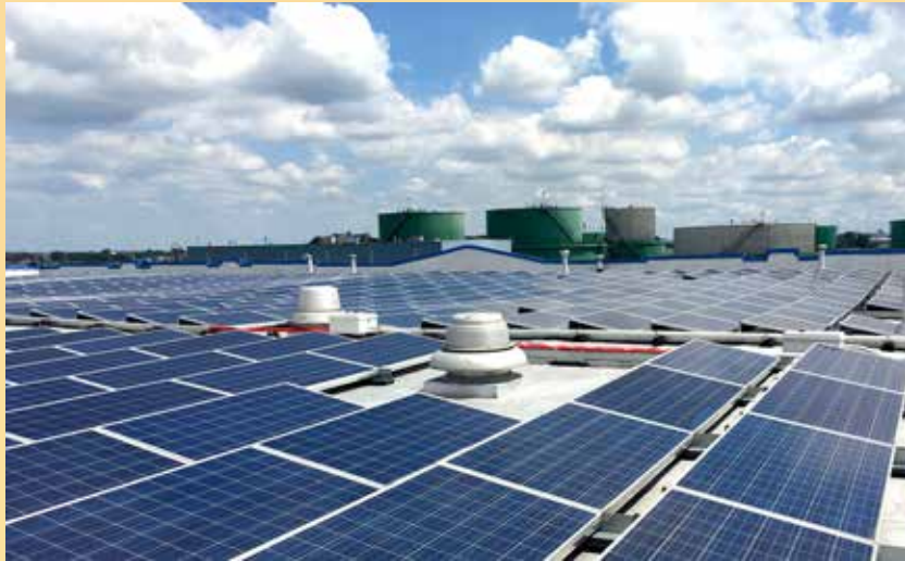
A 375kW community solar installation atop a warehouse in Bronx, NY. Photo by Travis Tench.
