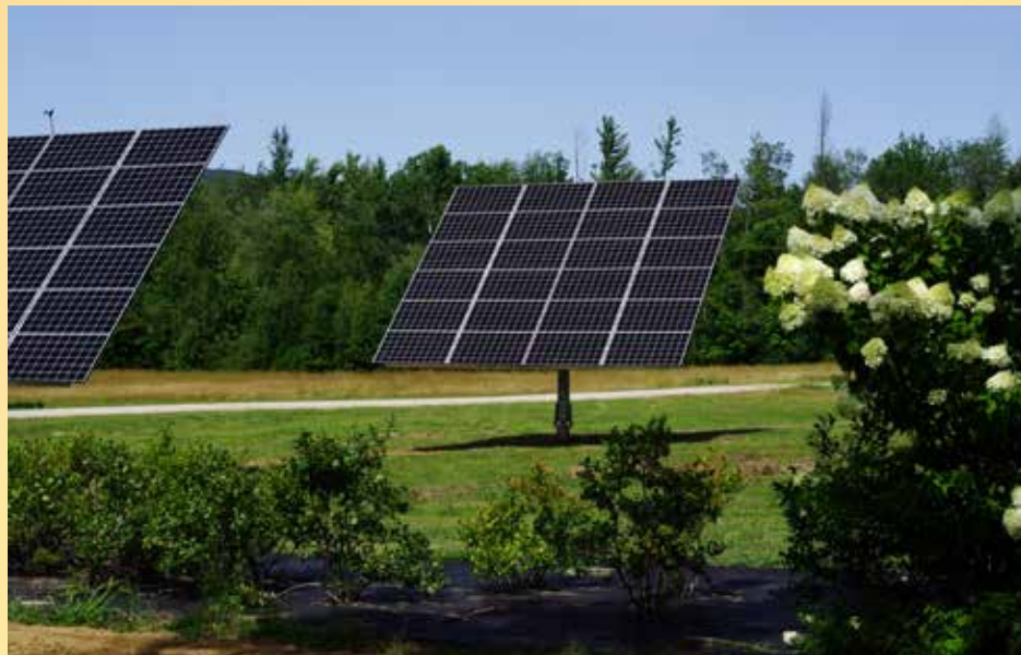
Solar trackers at Pooh Corner Farm. Photo courtesy of Maine Solar Solutions.
