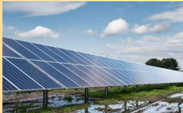
Above and at end: A 5.5MW project in New Windsor, NY. This is the largest community solar project in New York's Hudson Valley producing enough power for about 750 homes. Photo by Green Street Power Partners.
