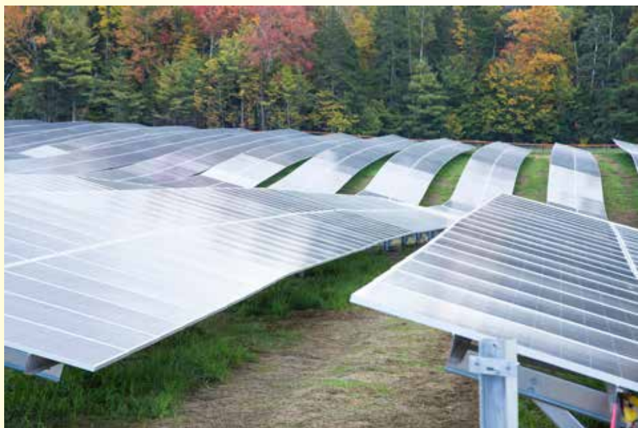
The Coolidge Solar Project, the largest solar array in Vermont, is 20MW and consists of about 83,000 photovoltaic panels. Image: NextEra Energy.
