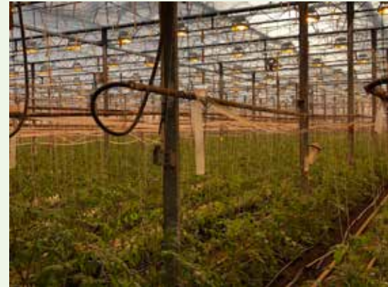
New greenhouse lights were installed at Long Wind Farm in Thetford, VT where tomatoes are grown all year. This project helps to reduce Long Wind Farm's carbon footprint. Image: GMP.
