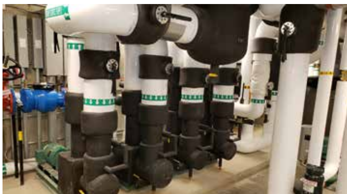
The Glen House has many pieces of hardware, including the geothermal circulation pumps seen here, that save money and energy. Image: Mt. Washington Auto Road.
