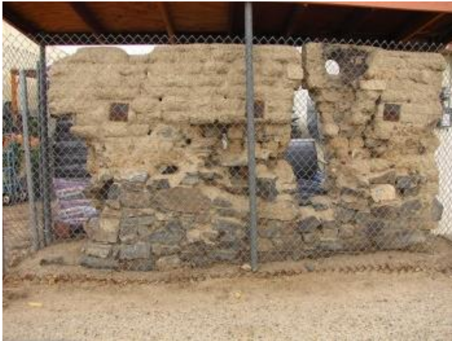
Adobe home damaged by 1872 Owens Valley Earthquake at Lone Pine. From https://www.sierranevadageotourism.org/images/otc/input/content/350/sieADC3FF3C413624523.jpg . Accessed June 23, 2019
