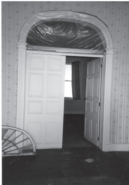
(right) One of the fine architectural elements of the Handy House is the fanlight window over a pair of paneled doors in the parlor. The window has been removed for repair in this photo, ca. 1990, by Bill Penn.
