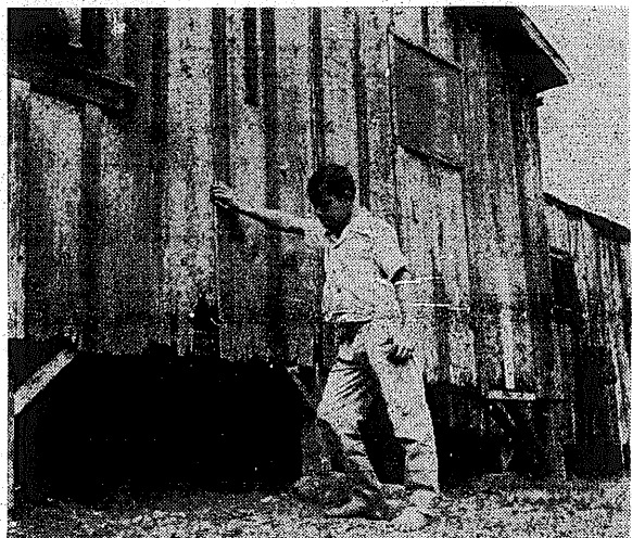
AFTER FIFTY YEARS the termites have almost nothing to chew on in this house, which is falling apart. "You can't punch the walls, even for fun," says a son of a tenant in an Aiea plantation camp, who is looking at a hole in the wall caused by the decaying, termite-ridden wood. Sanitation and precautions from fire hazards are unheard of in this camp.
