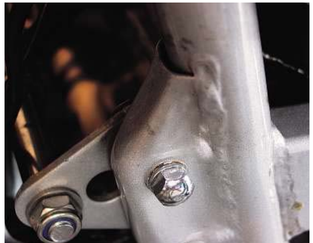
Gaps in welding can leave rusty streaks after powder coating.
