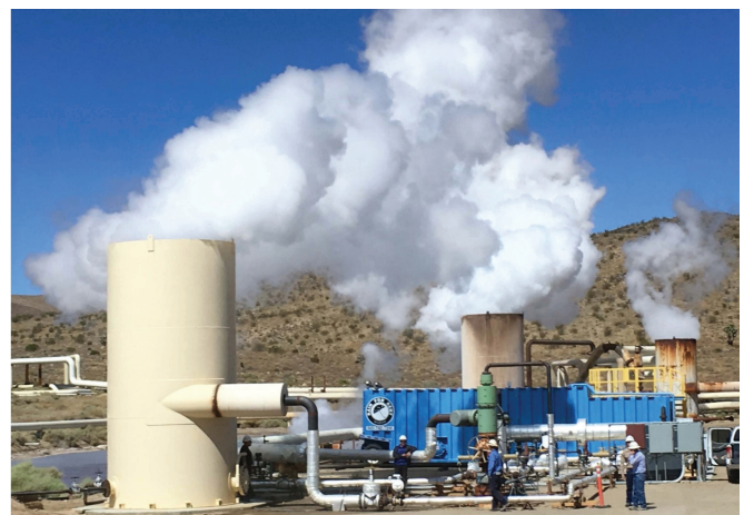
Figure 2. GreenFire Energy’s demonstration of a Closed-Loop Geothermal (CLG) energy system at the Coso, California geothermal power plant. September 2019.
