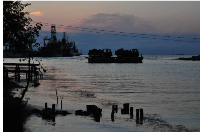
Starting harbour construction adjacent to the contested Kulevi oil terminal in the Kolkheti National Park Ramsar site, Georgia (photo: HJ 14-09-2012).
