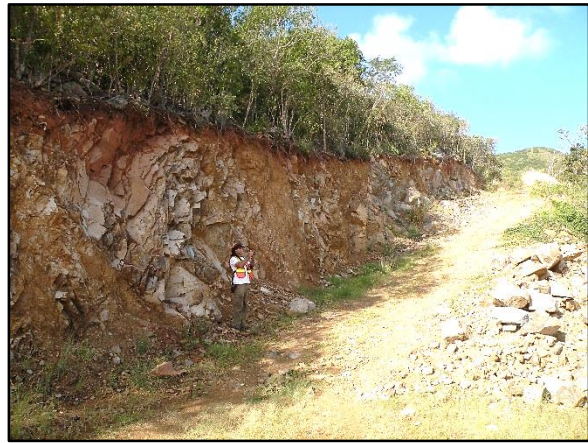
Photo 153. Typical "cut-and-fill" road construction along a steep slope on Tortola. The road cut face is approximately 6 m (20 ft) high.
