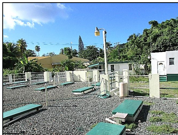
Photo 144. Sewerage treatment plant at Cane Garden Bay.
