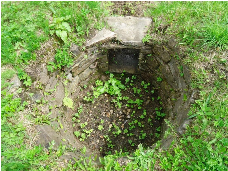
Plate 16. The roofless circular chamber of Mountallen sweathouse from a slightly elevated perspective. The north-east facing lintelled passage is in the middle background. (Image by the author).
