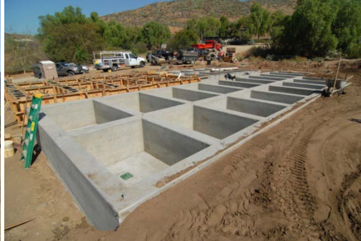
Foundation of Griffin Reptile Conservation Center showing individual cages and depth of each indoor/outdoor enclosure.
